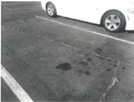
Photograph 13. View of surficial staining on asphalt located in the parking lot area on the subject property.
